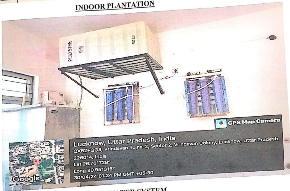
RO WATER SYSTEM
