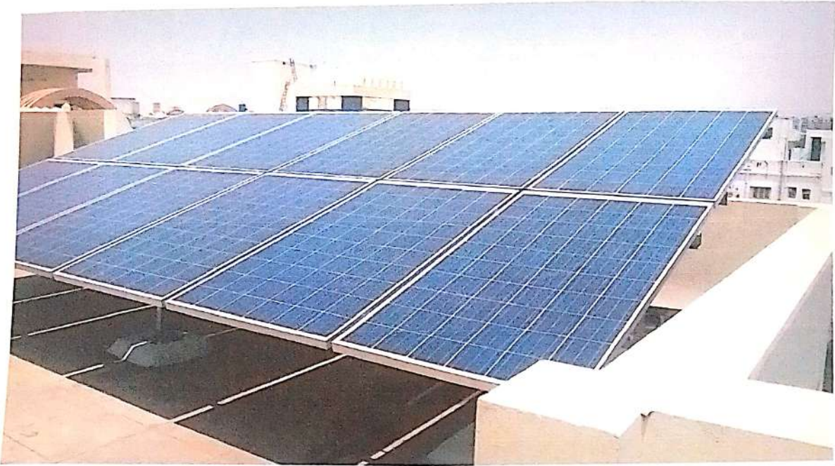
5KW on GRIDTIE SOLAR SYSTEM
